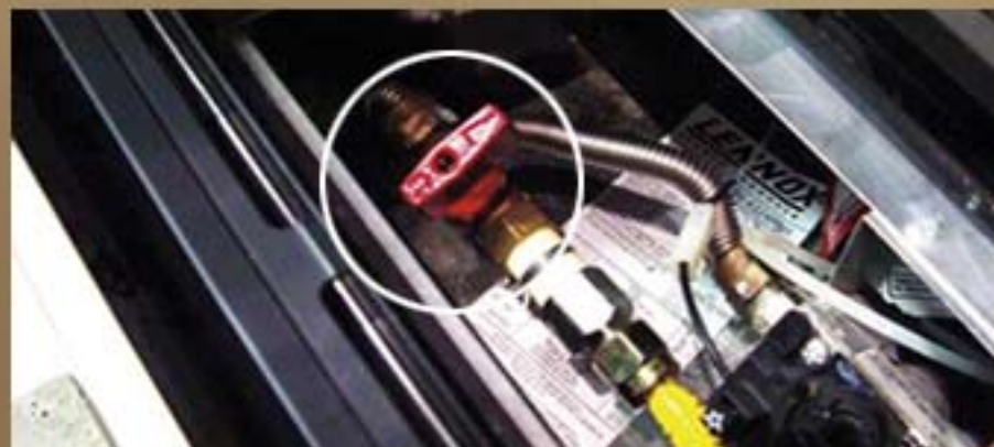
Gas supply in the OFF position
